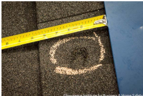
An impact is shown on one of the test specimen's impact-resistant laminate shingles. The majority of impacts on these shingles were only cosmetic.
