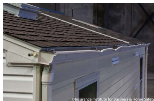
Damage to the test specimen's aluminum gutters.
